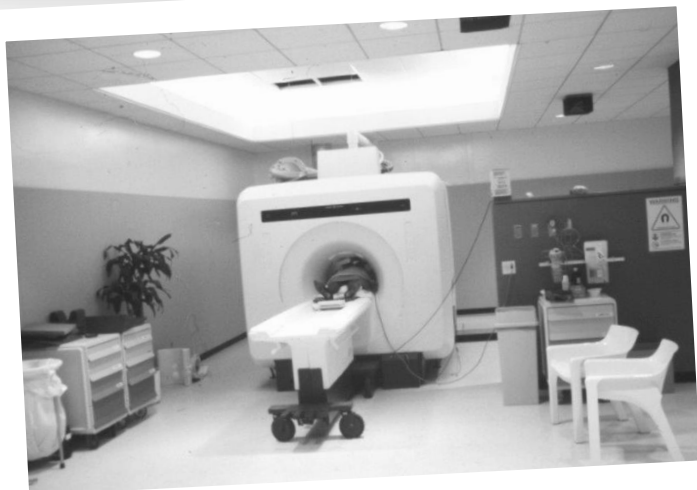
From top: 1986 MRI building courtyard, to facilitate delivery of magnet by crane as well as to provide protected space for magnetic field before magnetic shielding was available. MRI magnet during delivery. 1.5 Tesla GE MRI scanner, Room 1, MRI building.
